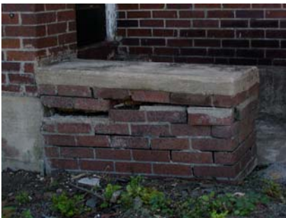
BRICK PILASTER IN NEED OF REPAIR
